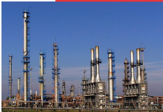
The MOL Algyő gas plant in Hungary
